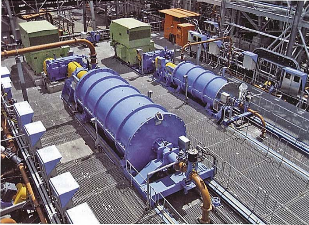
The Xstrata Technology M10,000 and a M3000 IsaMill that have been installed at Anglo Platinum's Amandelbult PGM concentrator in South Africa
