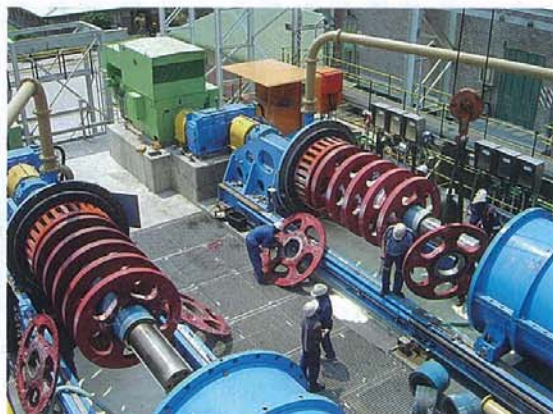
Maintenance on Anglo Platinum PPL A/B operation using 2 x M10,000 IsaMills. The initial mill was designed with a 3000 L grinding chamber.
