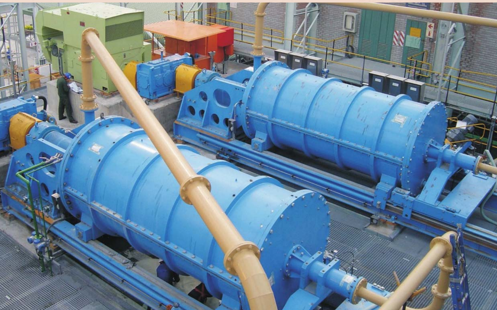
Installation at MSC A and B.
