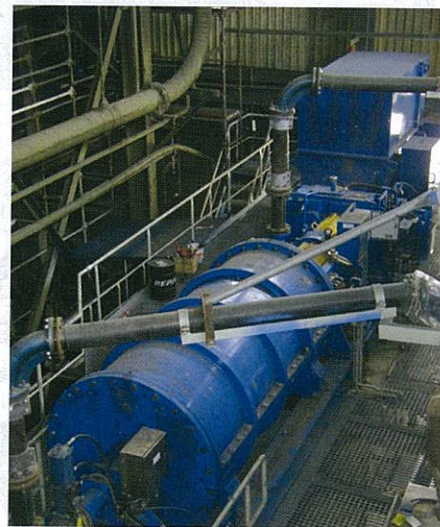
The 500kW IsaMill M1000 is part of the lead regrind circuit that is required to liberate the lead rougher concentrate at the Neves-Corvo operation in Portugal.
