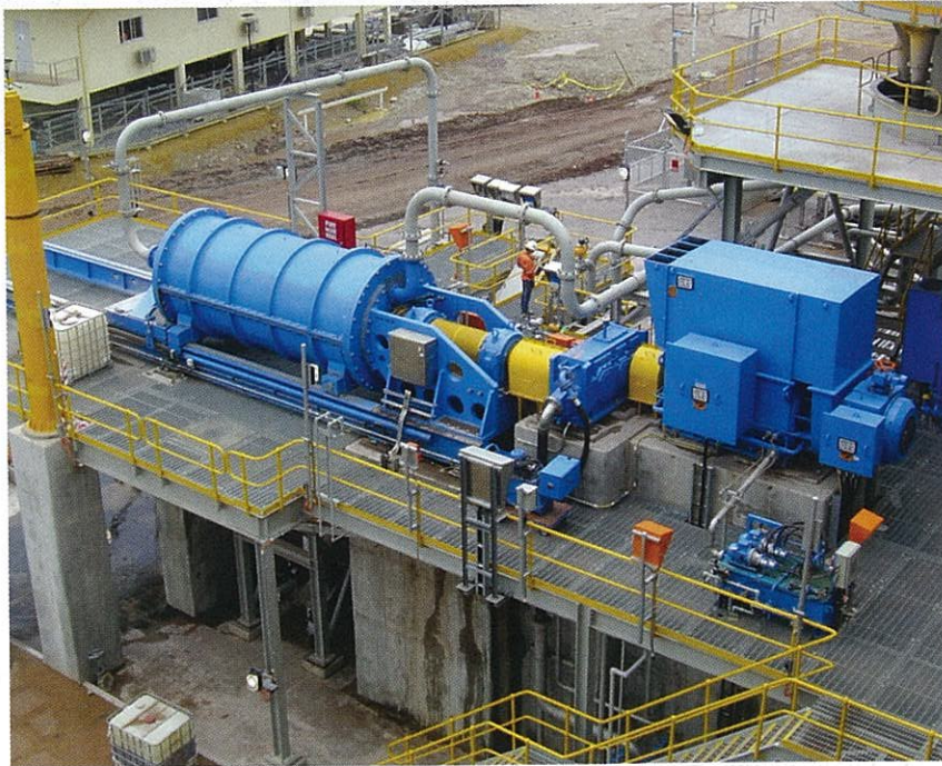
This 3,000-kW M10000 IsaMill was installed at PanAustrian's Phu Kham copper operation in Laos in 2007. In October 2010, the company approved a $110-million investment to increase capacity of the Phu Kham process plant to annual copper production of 65,000-70,000 mt starting in mid-2012. The scope of the upgrade includes an increase to a nominal 16 million mt/y of ore from the current rate of 12 million mt/y.
