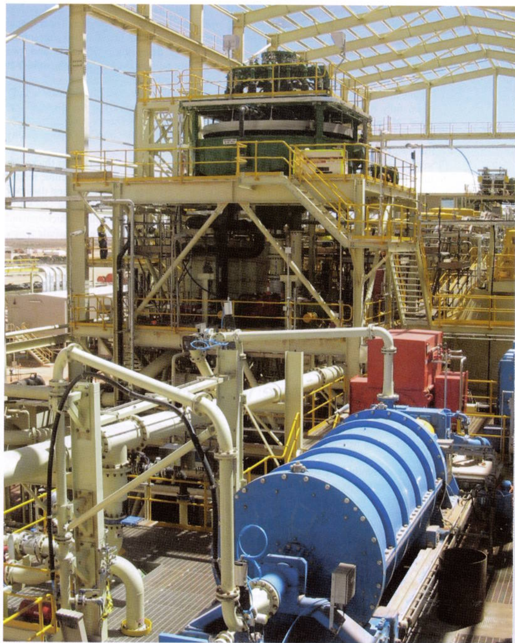
The IsaMill and Jameson Cell at Prominent Hill has been married to conventional float cells to get high recovery in a small space.
