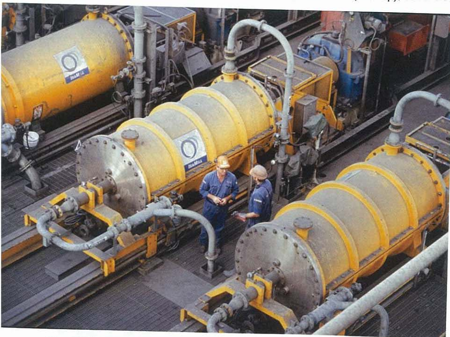
The M3000 IsaMills are powered by 1500 kW (2010 hp) motors.
