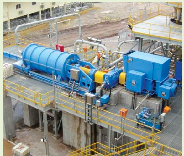
M10,000 IsaMill™ operating at the Phu Kham operation, Laos. Commissioned in 2008, the mill operates with MT1™ ceramic media, and operates in the copper gold regrind circuit.
