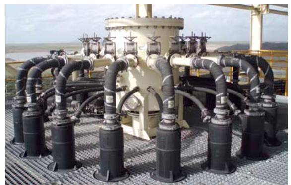
Mark IV Jameson Cells installed at Lake Vermont, Australia
