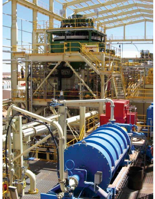
The 3MW, 4000HP, M10,000 IsaMill™ and B5400/18 Jameson Cell installed in the flotation circuit at the Prominent Hill copper-gold concentrator, South Australia
